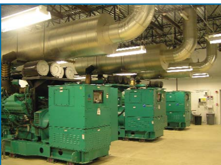
Generators provide back-up power to the Hospital during area power outages.
