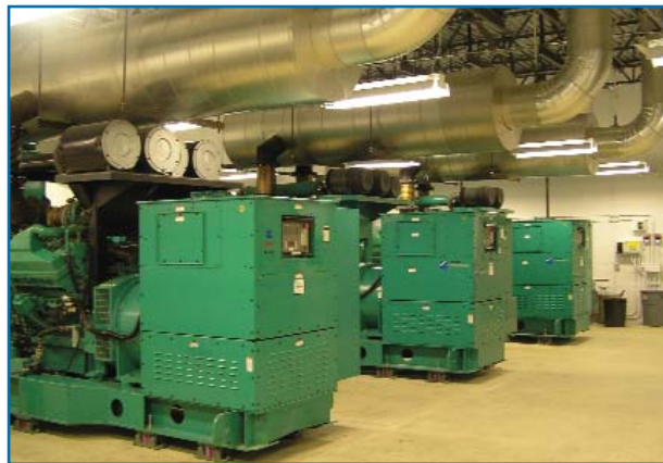
A recently installed back-up generator system in place as of fall 2004 allowed Licking Memorial Hospital to not miss a heartbeat during a widespread holiday-time power outage in Licking County.
